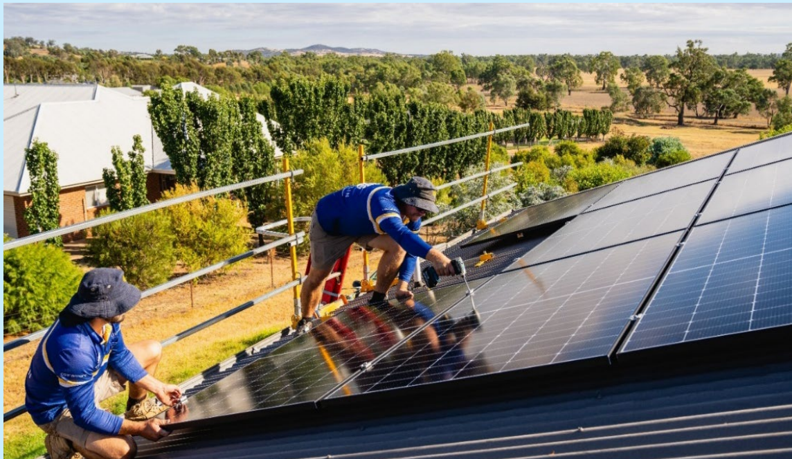
Figure 8: Rooftop solar installation. Source: DCCEEW
