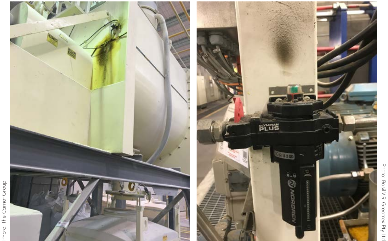
Figure 12: Examples of compressed air leaks that impact surfaces, with entrained dust particles forming a smudge or line on the same surface
