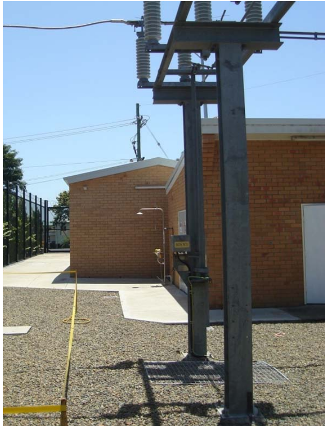
Figure 4 - Tape is supported by Stands, NOT High Voltage Structures
