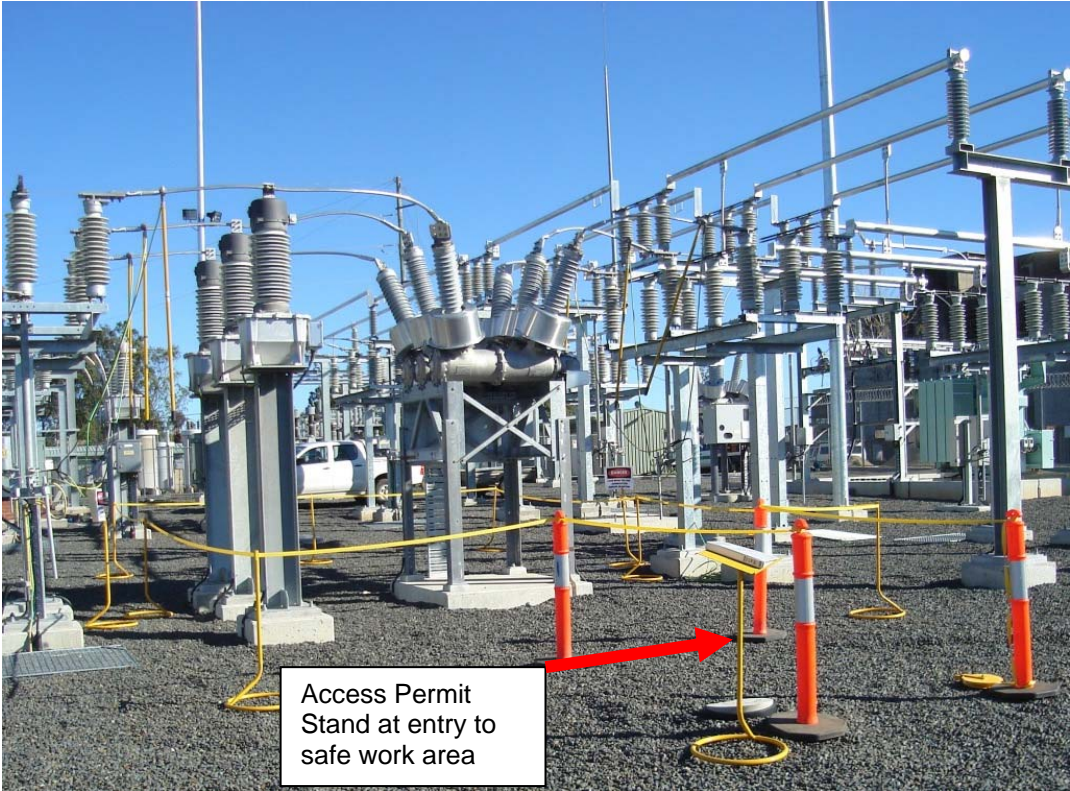
Figure 3 – Correct Safe Work Area Established for a Circuit Breaker Bay
