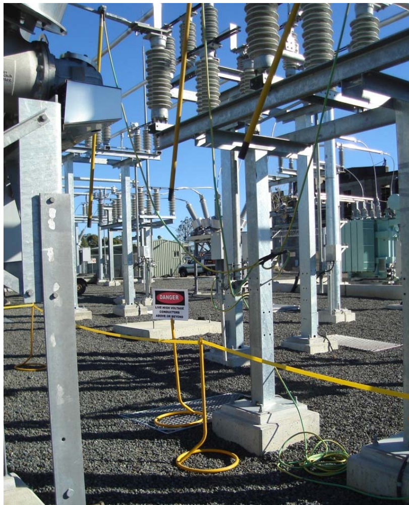
Figure 7 – Example of use of Danger Sign
