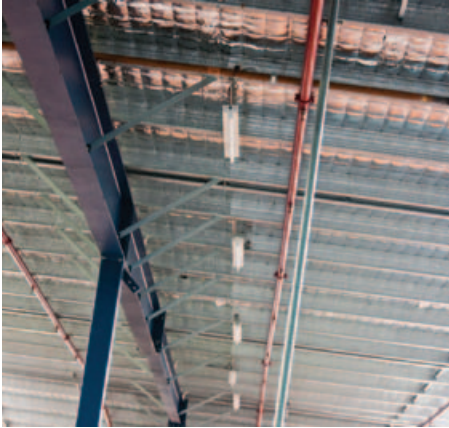
Figure 64: A row of single T8 fluorescents being used for emergency lighting
