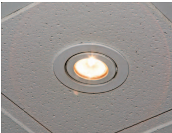
Figure 36: An existing halogen downlight
