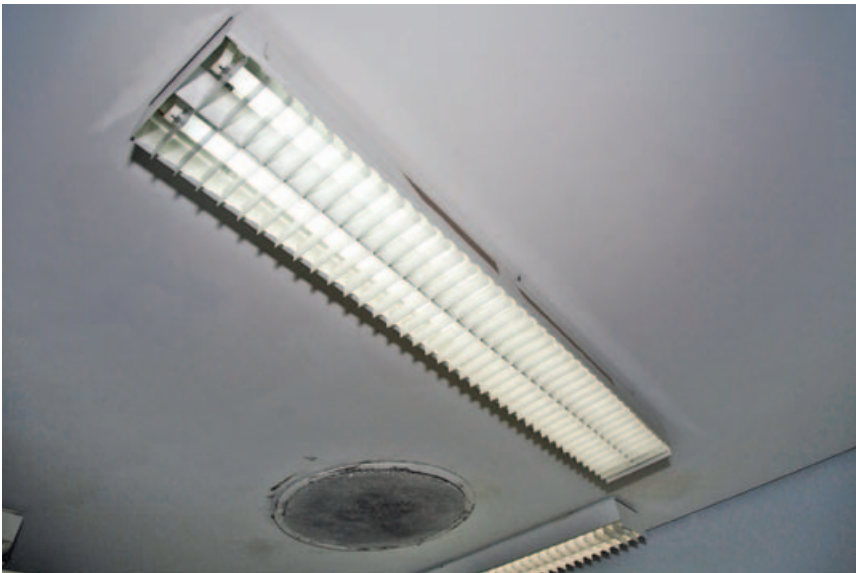
Figure 17: Twin T8 louvre lamps
