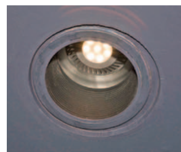
Figure 47: LED PAR lamp in a recessed downlight
