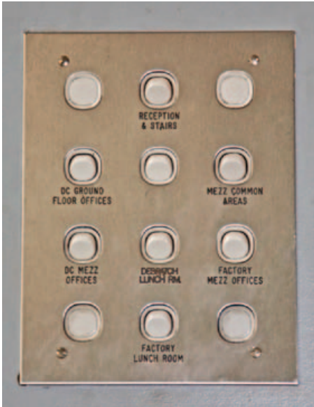
Figure 66: Light switch control panel
