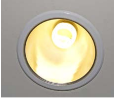
Figure 45: Compact fluorescent replacement lamp in a recessed downlight that was designed for a GLS lamp
