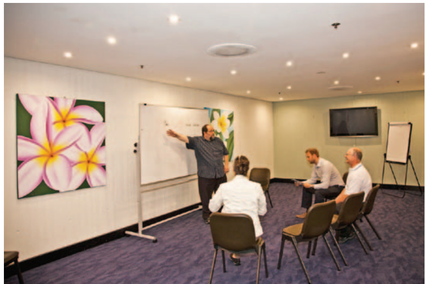
Figure 43: A meeting room with new LED downlights replacing old halogen lights
